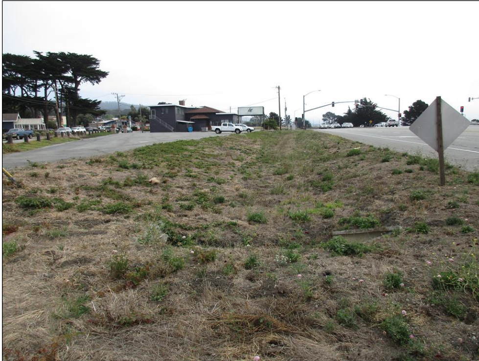
Photo 5: View looking south from the northern end of the drainage swale location on the north side of Cabrillo Highway. Photo shows the culvert inlet which conveys water beneath the highway to the drainage swale on the northeastern edge of the Project Area.
