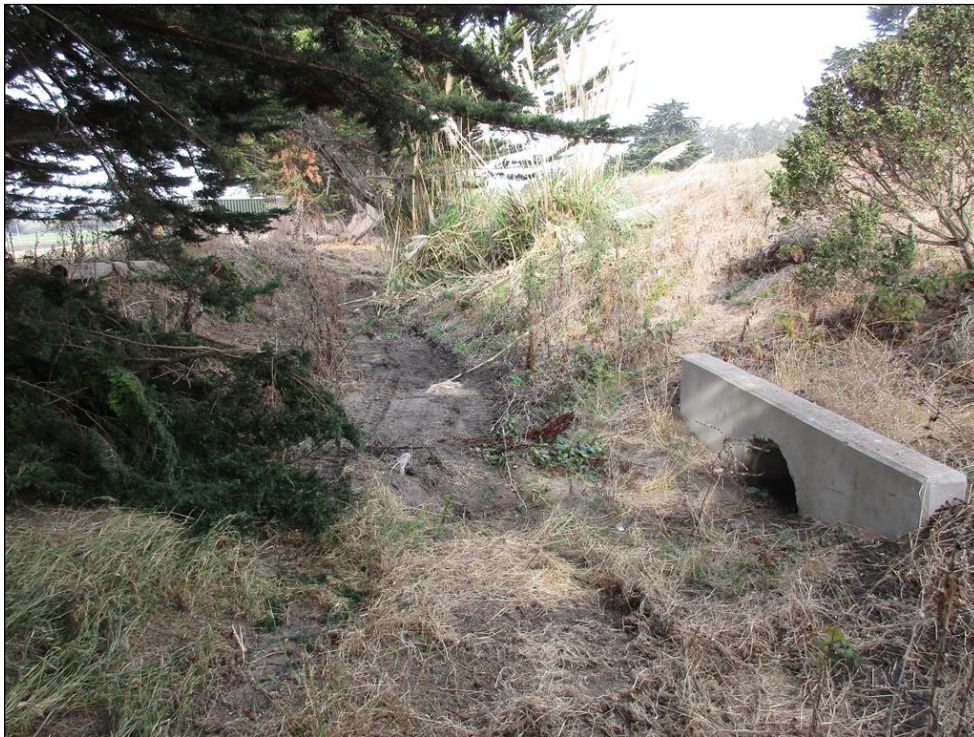
Photo 4: View looking northwest along the ephemeral drainage swale along the northeastern boundary of the Project Area. Photo shows the location of the culvert outlet which conveys water from the north side of Cabrillo Highway to the drainage swale.
